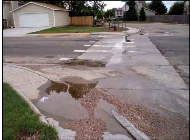
Figure 29. Some curb ramps near Dildine Elementary School are in poor condition
