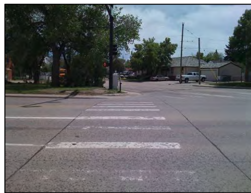
Figure 9. Faded crosswalks can be hazardous to pedestrians
