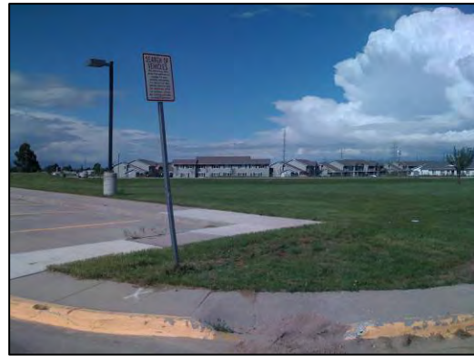
Figure 12. Curb ramps with steep grades, and/or poor maintenance can render a sidewalk inaccessible to a pedestrian in a wheelchair
