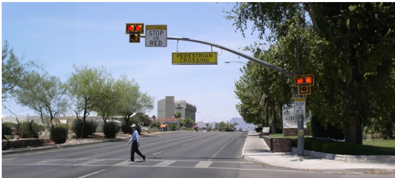
Figure 48: Crossing signal (Credit: Michigan Complete Streets Coalition)
